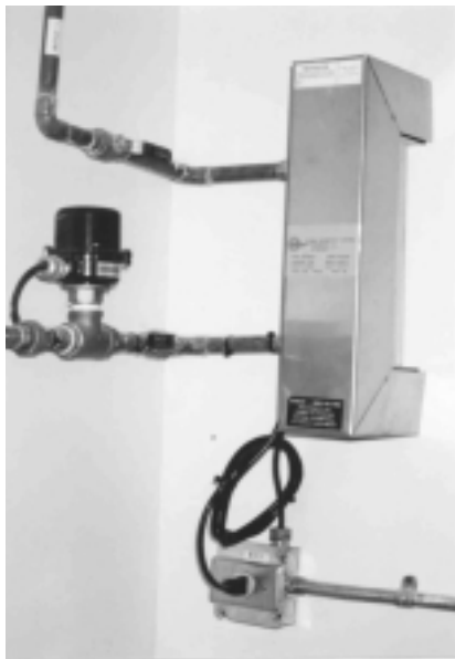
Flow switch and ultraviolet water purifier
