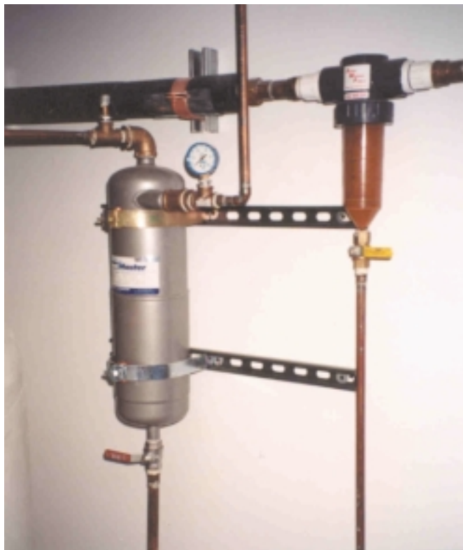
Sand filter and tank pre-filter
