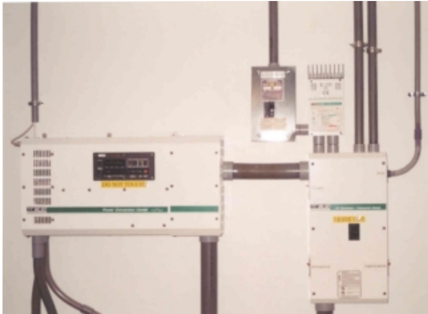
24-volt DC to 120-volt inverter and solar battery charger
